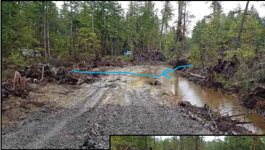
Photo 7: View on opposite side of road alignment. Pondered water along road at upper end of the Middle Stream side channel; Southern half of property.
