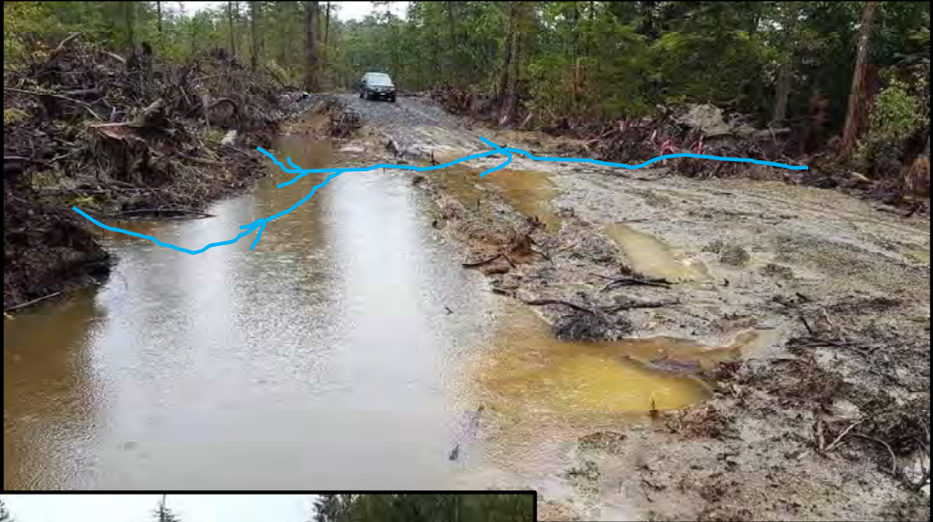
Photo 8: Impacted drainage. Area to be integrated into stormwater management plan for site. Overflow from the Middle Stream in the southern half of property.
